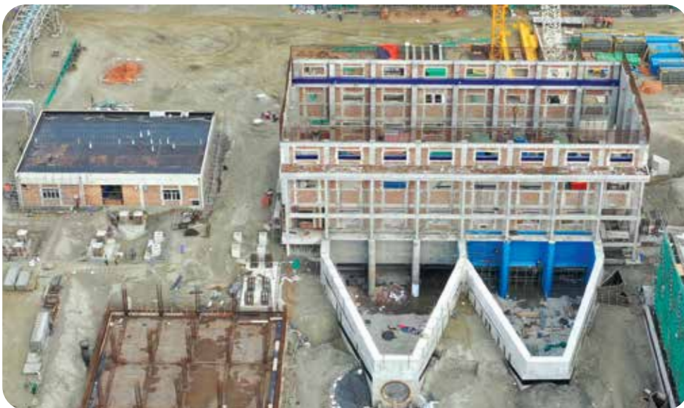
CW Pump Station : Payra 1320 MW TPP Project (1st Phase)
