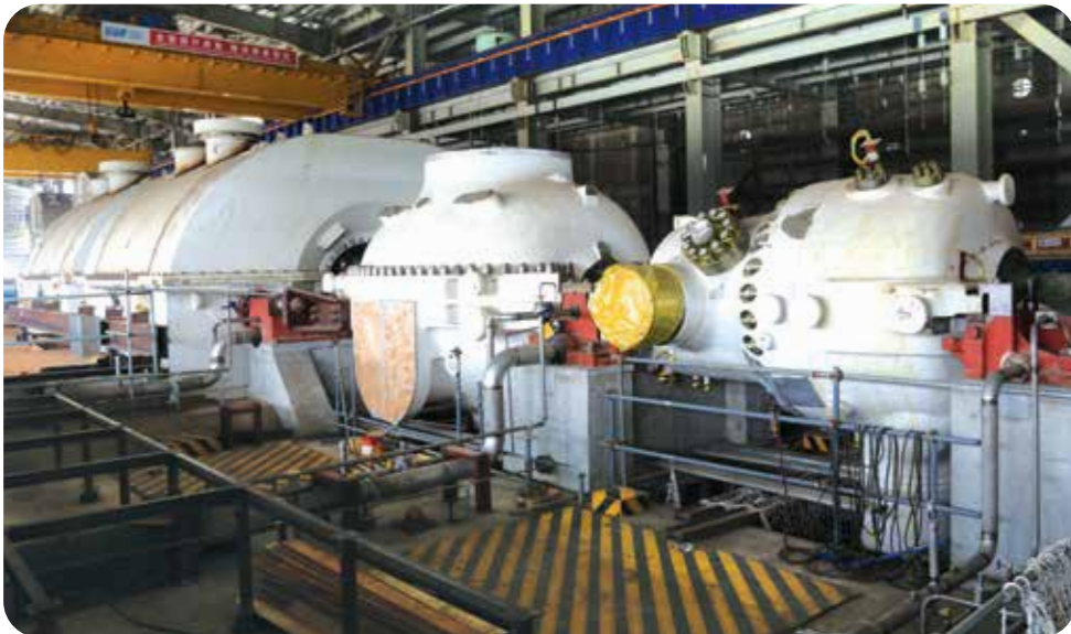
Turbines: Payra 1320 MW TPP Project (1st Phase)
