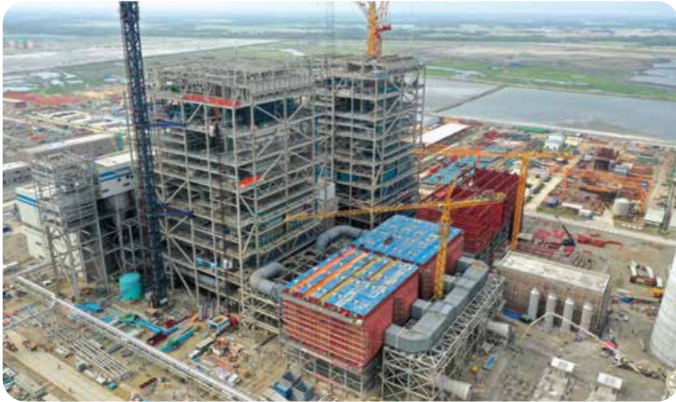
Boiler Unit 1 & 2 : Payra 1320 MW TPP Project (1st Phase)
