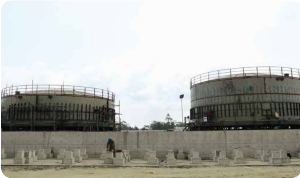
Fuel Tank : Payra 1320 MW TPP Project (1st Phase)
