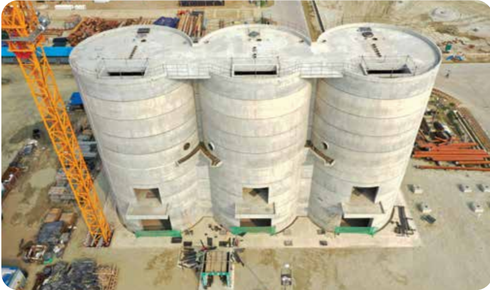
Fly Ash Silo : Payra 1320 MW TPP Project (1st Phase)
