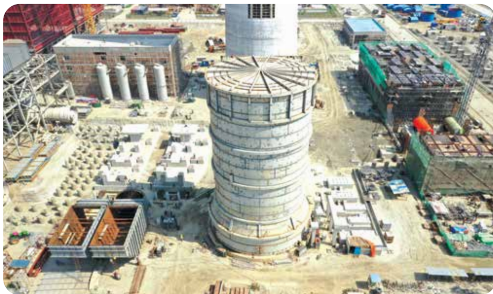
Absorber : Payra 1320 MW TPP Project (1st Phase)
