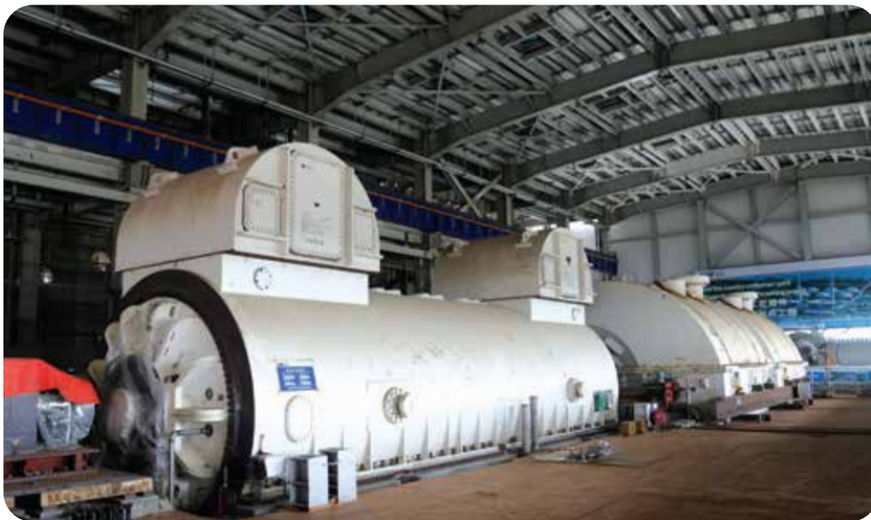
Generator : Payra 1320 MW TPP Project (1st Phase)
