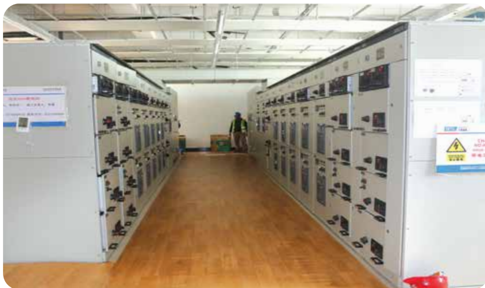
Switchgear Room : Payra 1320 MW TPP Project (1st Phase)
