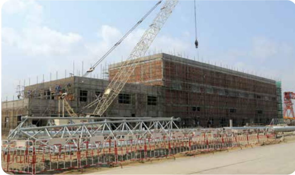
400 KV GIS Substation : Payra 1320 MW TPP Project (1st Phase)
