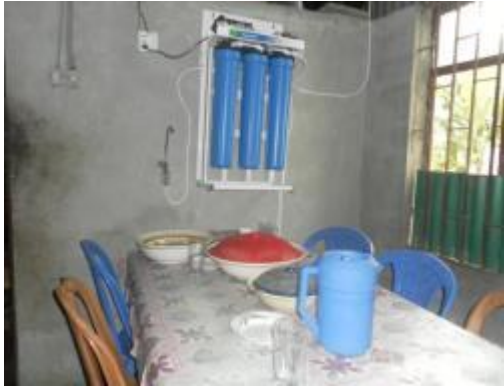
Water Treatment System For NDE Labors
