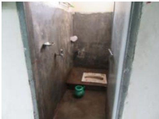
NDE Employees' Toilet Facilities
