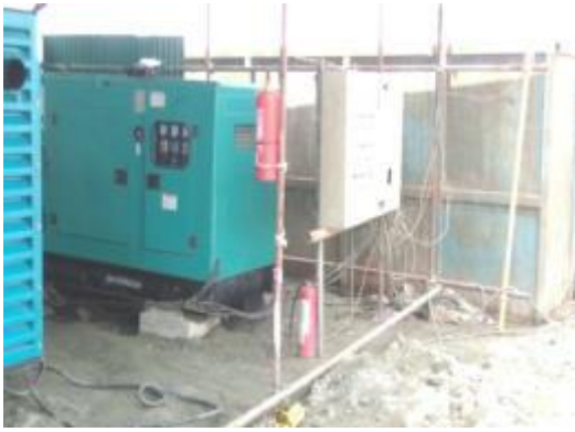
Fire Extinguisher in Project Site
