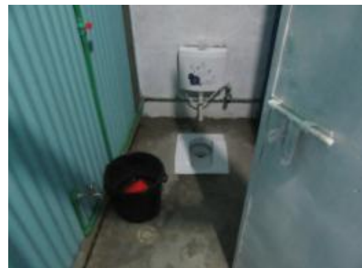
Toilet facility (NEPC)
