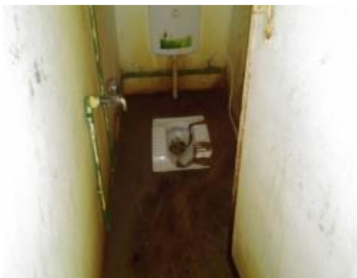
Irregular Cleaning In NEPC Subcontractor Labors' Sheds
