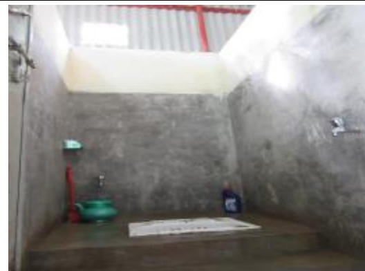
NDE Employees' Labor Shed Sanitary Conditions
