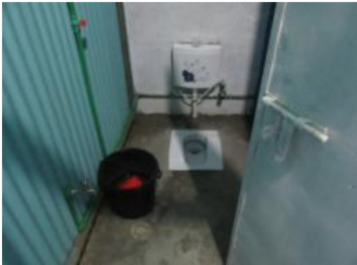
Toilet facility (NEPC)
